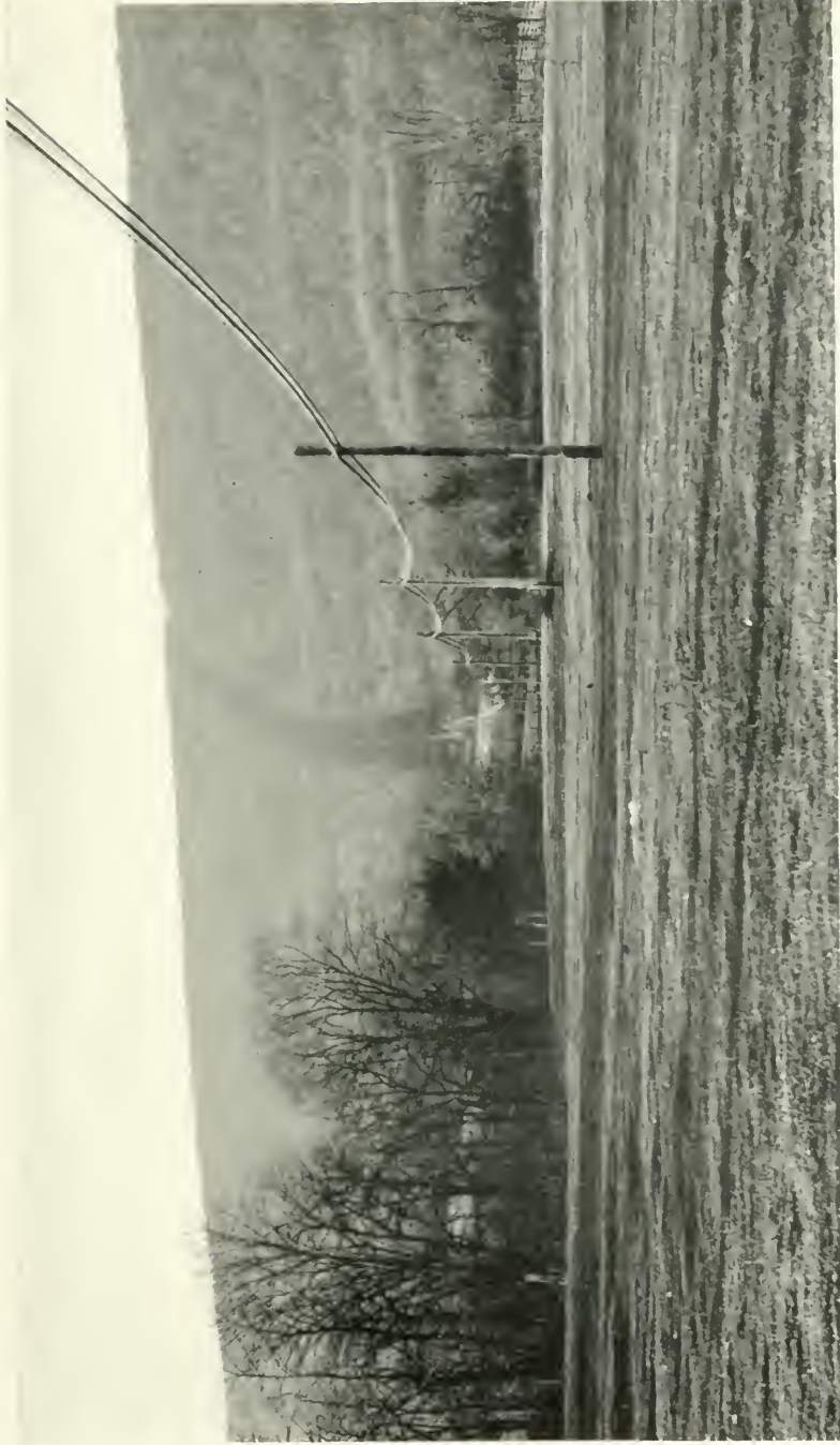
FIGURE 5. TWO CABLES ON ONE OF THE HARRISBURG-PITTSBURGH ROUTES. THIS ROUTE IS THROUGH BEDFORD.
